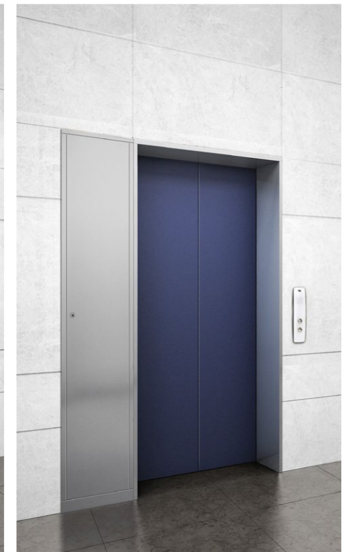
Entrance with control panel
